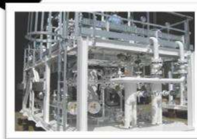
Fuel Gas Conditioning Unit for 15MW Power Plant RM24m
